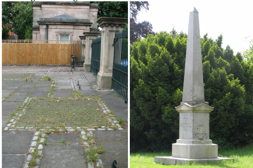
(Left) Weeds growing through paving adjacent to the Norman lodge; (right) graffiti and damage to the Jackson Memorial.
