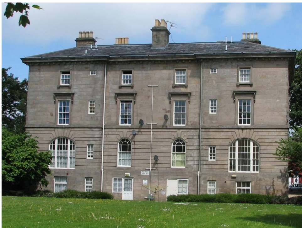
The effects of multiple occupancy on the park-facing side of Roden House. There are additional waste pipes, vent pipes through the roof, a number of satellite dishes and signage on the building.
