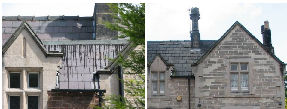
(Left) The photograph shows an example of a particularly poor quality repair that is severely detrimental to the appearance of a listed building. The bitumen used to adhere the felt over the ridge (in itself detrimental to the building) has dripped down over the slate, almost certainly cause irreparable damage. (Right) Excessive and probably unnecessary mortar repairs of the face of the stonework.
